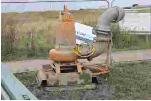
One of 5 electric driven water pumps
