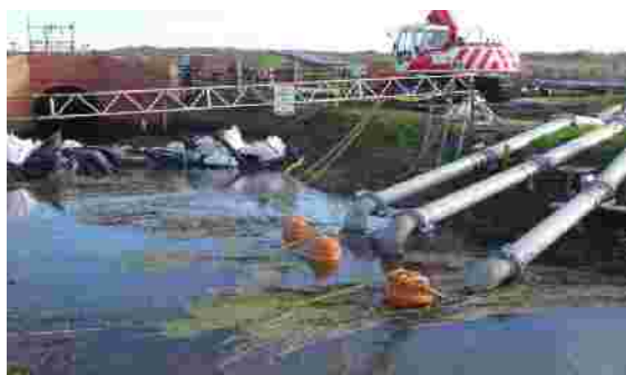
Three pumps working under flood conditions
